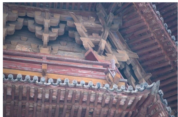
Figure 4: Dougong system constructed on the Yingxian Wooden Pagoda. Screenshot from The Preservation of the Yingxian Wooden Pagoda (Lai, 2018).
