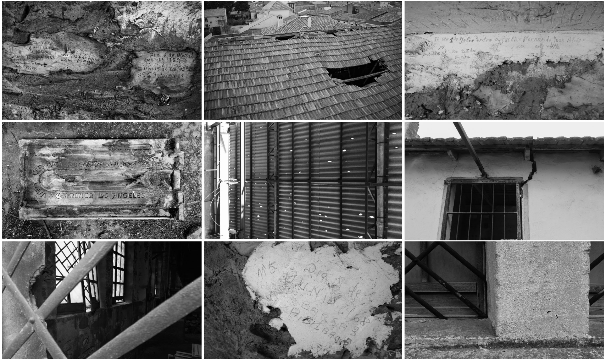
Fig 24. Taller dels Canets (former San Antonio wooden carriage factory), Beneixama (Alicante, Spain), January 2021. Exterior photographs in detail of the workshop initial state before measurements and drawings were made. Materials, texture, surfaces. (Ortin Molina, S.; Ortin Molina, M. A., photographs and digital image post-editing work).
