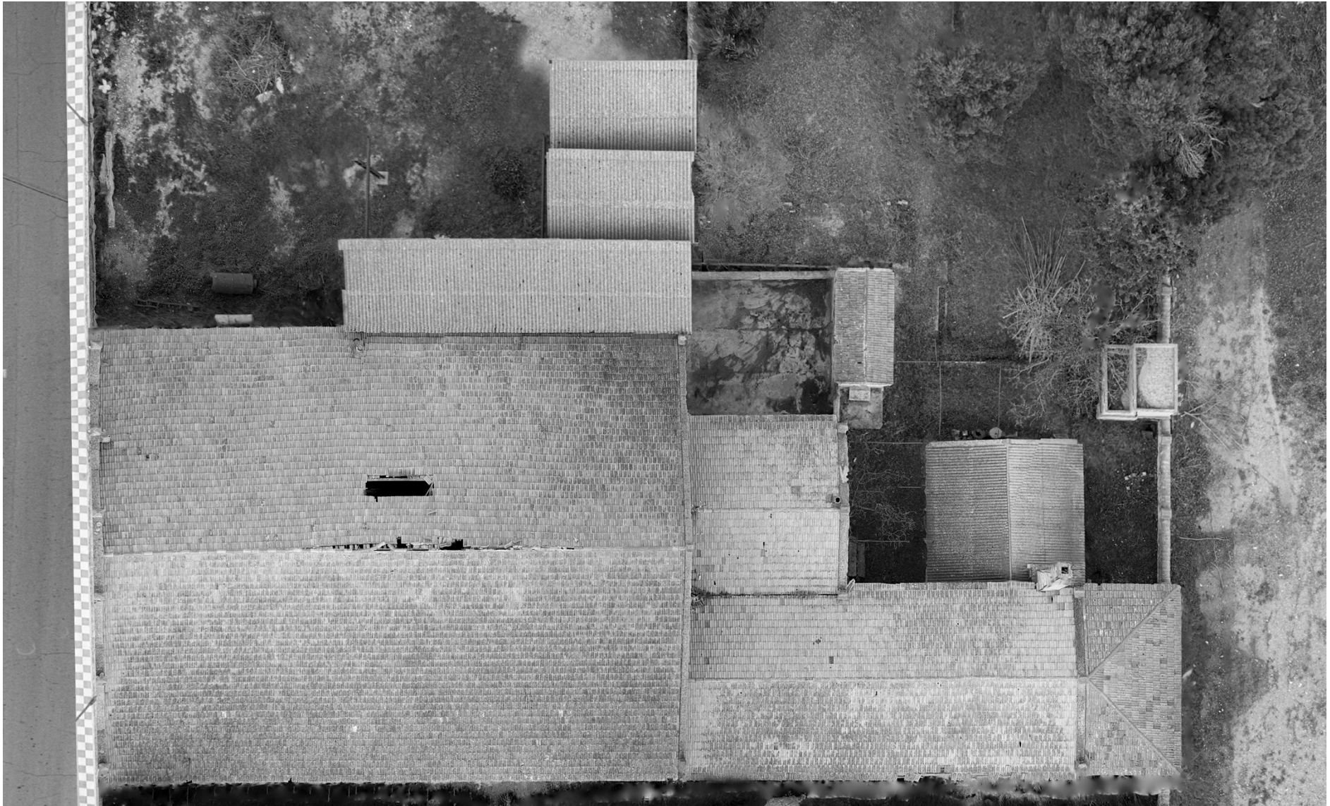
Fig 6. Taller dels Canets (former San Antonio wooden carriage factory), Beneixama (Alicante, Spain), April 2021. Aerial photography taken with drone of the current state of the workshop. The roof is seriously damaged as a result of the last snowfall in 2019. (Courtesy of Martínez Pérez, A. (Arqueojocs); Molina Carbonell, J. (MuixegoDigital)).
