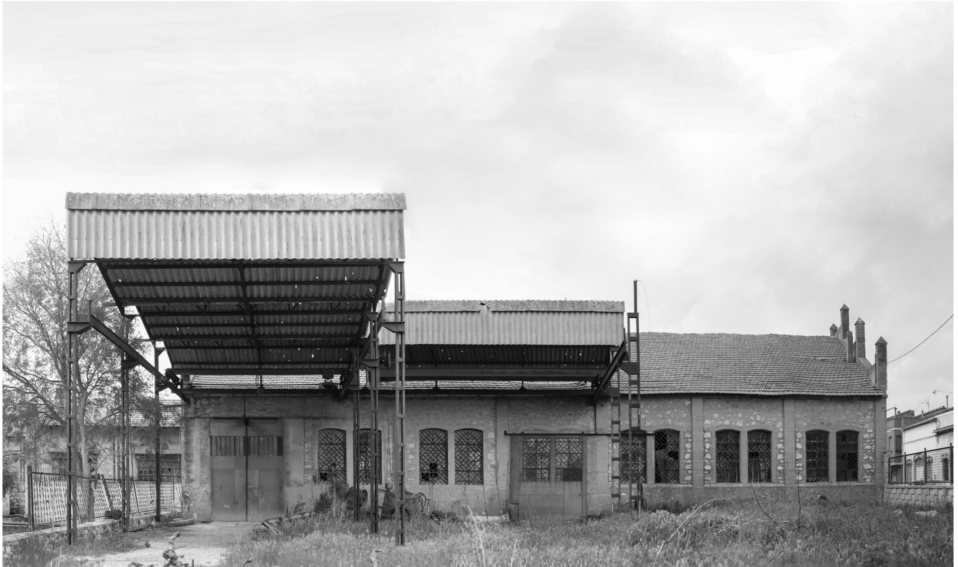
Fig 19. Taller dels Canets (former San Antonio wooden carriage factory), Beneixama (Alicante, Spain), April 2021. Exterior photograph of the workshop main nave east elevation. The decay of the annexed outer space, completely abandoned to nature. (Ortin Molina, S.; Ortin Molina, M. A., photography and digital image post-editing work).
