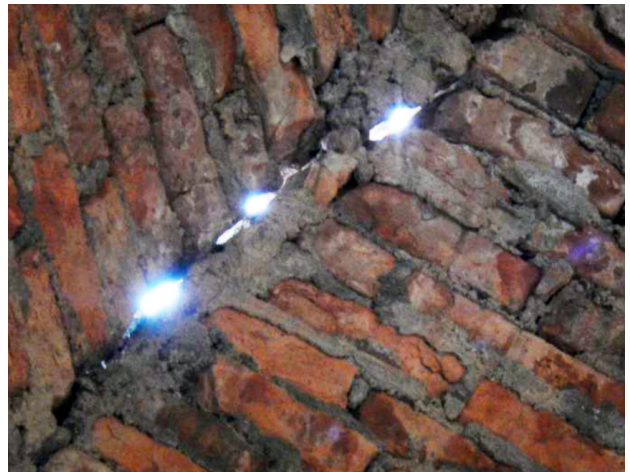
Figure 9. Fissures on caskets of the dome of the temple of Santa Lucía. Source: by the authors
