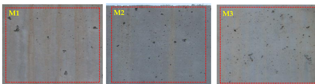
Figure 6. Three concrete walls analyzed (M-1, M-2 and M-3, from left to right).
