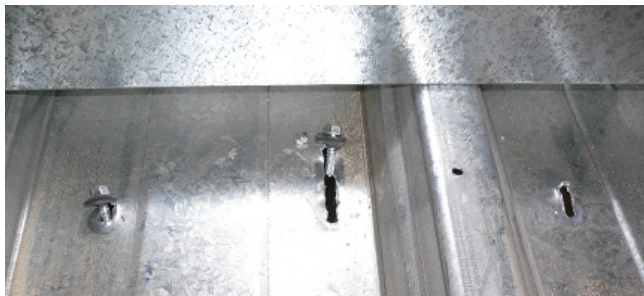
Figure 13: Tears caused by crushing of the steel sheet against the bolts in the supports.
