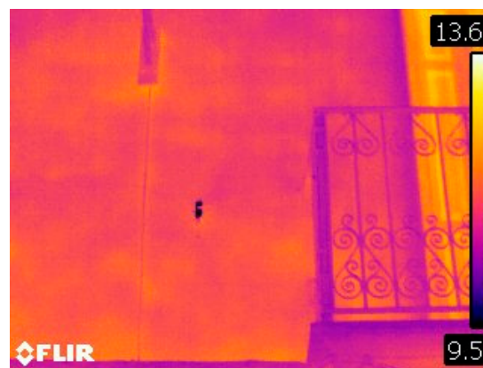
Figure 2. Verification with a thermographic camera of the wall surface with a datalogger. Source: L. Balaguer.
