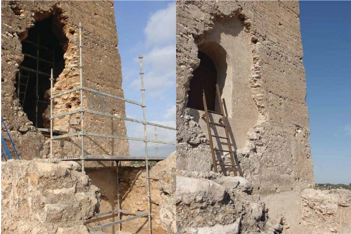
Figure 7. Reintegration works respecting the detail without having an impact on the overall view of the building (Cristini).
