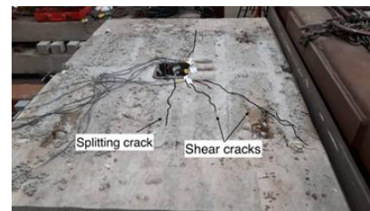
Fig. 10. Cracking pattern of slab of SP5
