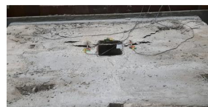
Fig. 12. Shear cracking of slab of specimen SP6
