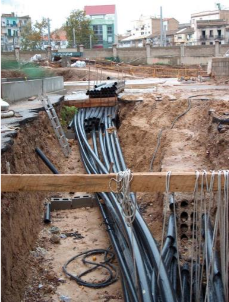
Figure 1. Placement of utility services underground is not generally accomplished in any systematic manner resulting in a veritable maze in high density urban areas
