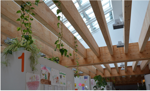
F132 Detail of plants in the multi-purpose space of Itoi Elementary School.
