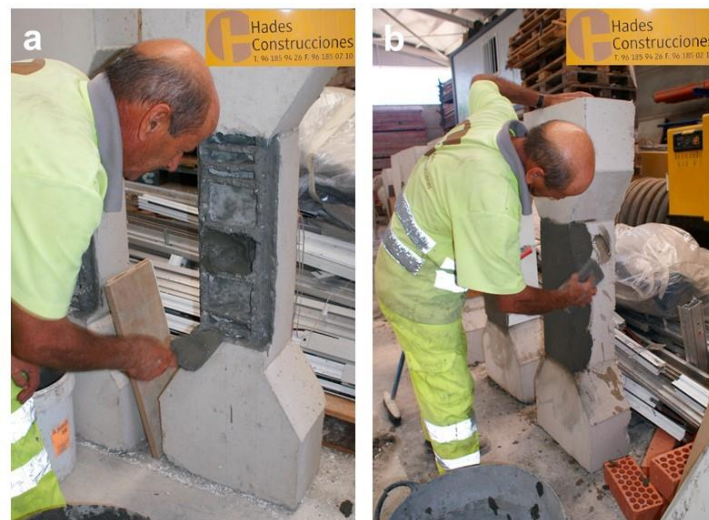
Fig. 4. a) Placing the first layer of the repair mortar; b) Smoothing the surface.
