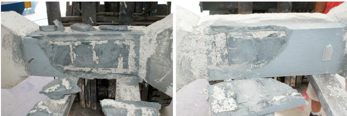
Fig. 11. Failure patterns in specimen B4. Detachment of a mortar layer
