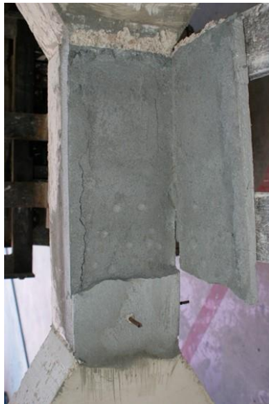
Fig. 9. Failure pattern in specimen W3. Detachment of a mortar layer
