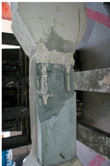
Fig. 7. Failure pattern in Specimen B3. Detachment of a mortar layer
