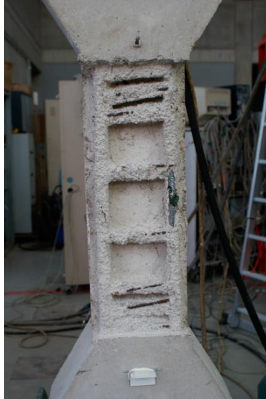
Fig. 6. Failure pattern in specimen D (damaged unrepaired columns). Buckling in rebars in side 3.
