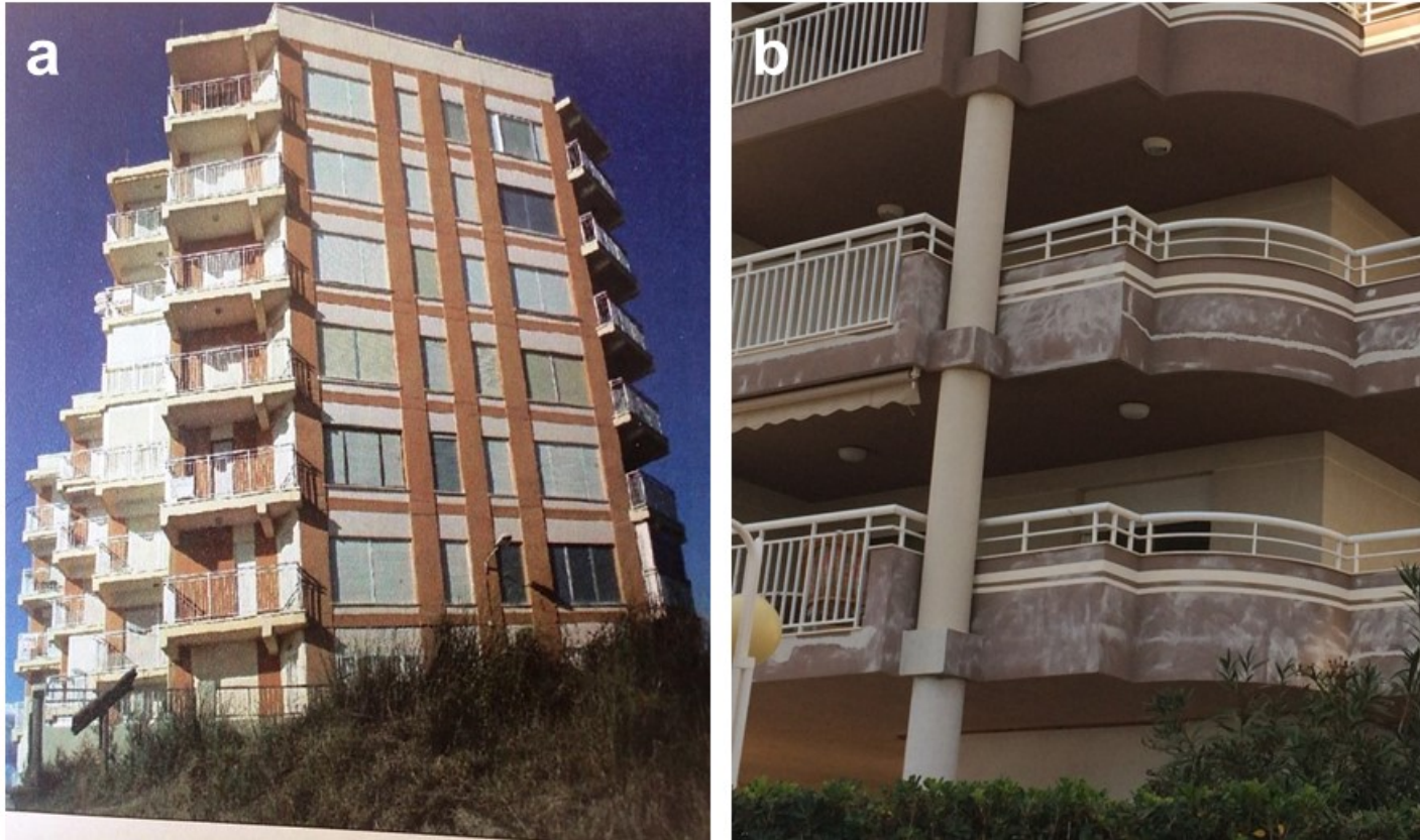
Fig. 6. a) Façade with mortar cladding, fronts of slabs, ledges and balcony beams with no protection (Cullera); b) Columns with painted cement-mortar rendering (Benicassim)
