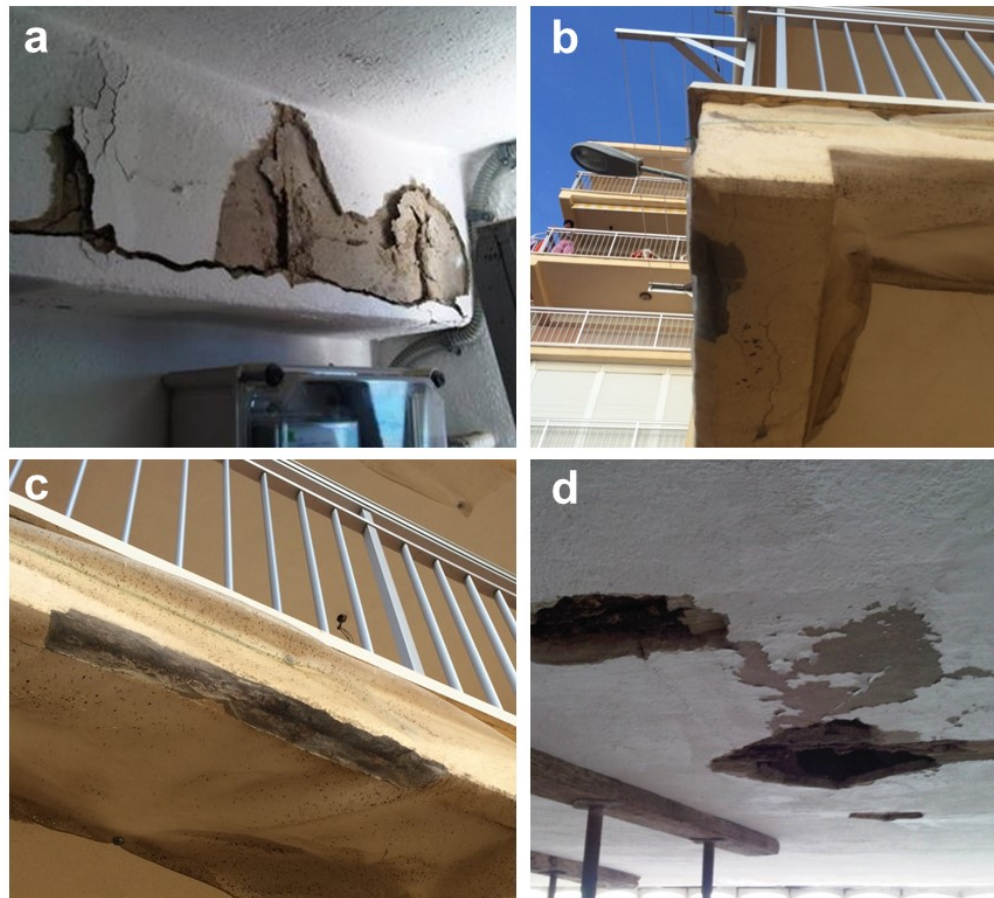
Fig. 4. Different damages in apartment buildings located in Valencia coast
