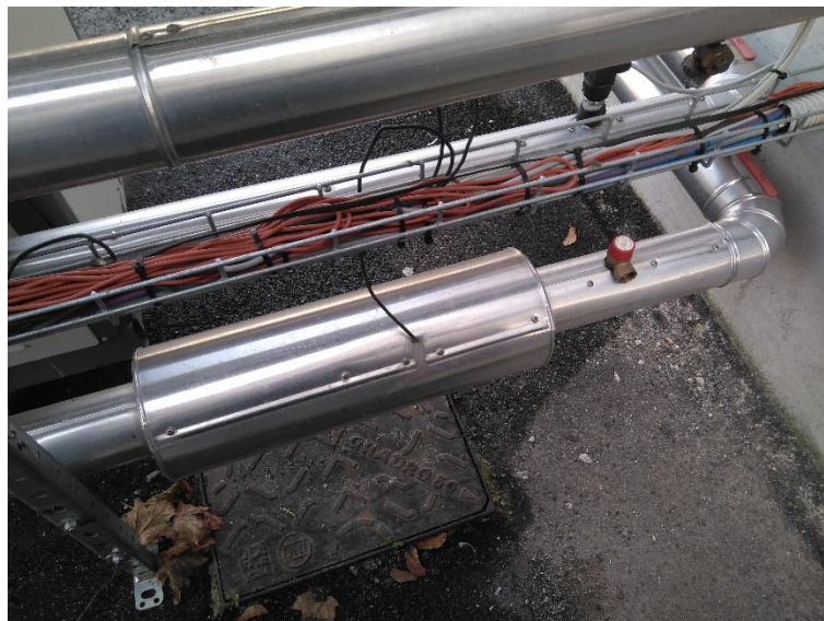
Figure 2.9. Flow meter (magnetic)
