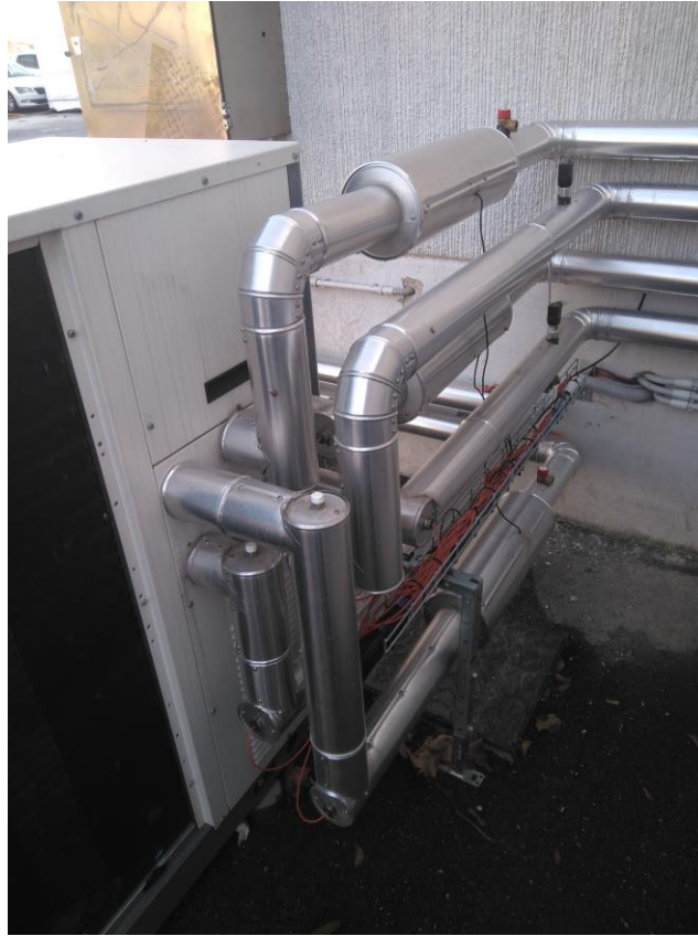
Figure 2.15. Back side of the DSHP unit: connecting pipes and sensors
