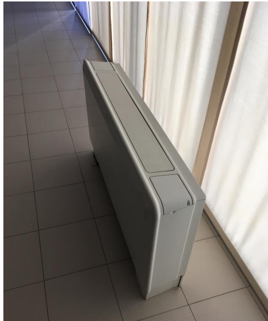
Figure 2.13. Fan coil Galletti FLAT S-20 installed in the meeting room
