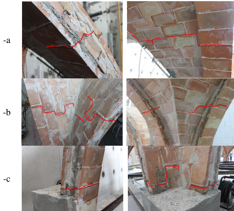
Figure 10. Cracks close to supports S1 (-a), S2 (-b) and S3 (-c).
