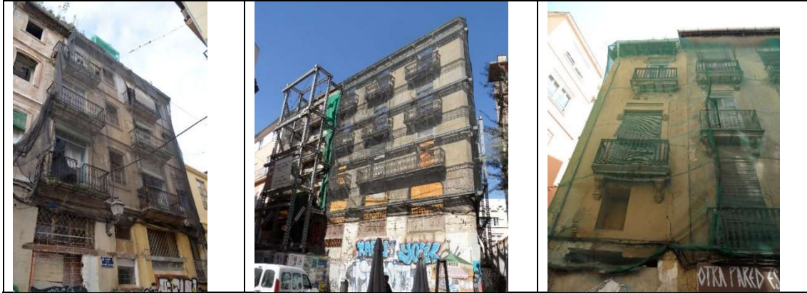
Fig. 3 Ruined buildings in Ciutat Vella (credit: the authors)
