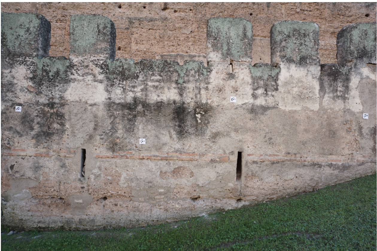
Fig. 8. Photograph of part of the outer barbican where some coded targets can be seen (Source: the authors).
