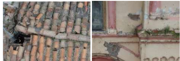
Figure 14. Damages in the church of Nabón
