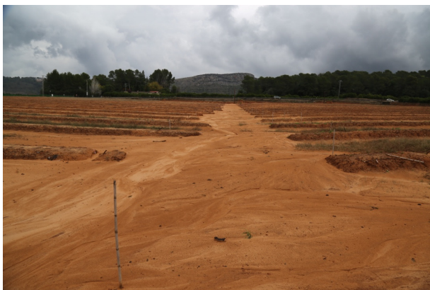
Figure 1: Soil erosion rates in Carcaixent (Spain) due to the plantation of new citrus crops. During the plantation works the soil is bare and soil erosion rates reach high rates. November 2019.
