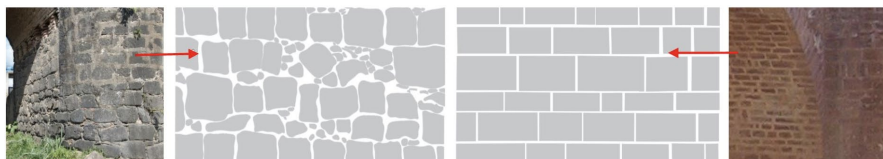
Figure 7. Left, masonry stone system of Los Esclavos Bridge. Source (Author 2018) Right, Masonry stone system of Las Donadas Bridge. Source (Garcia 2008)
