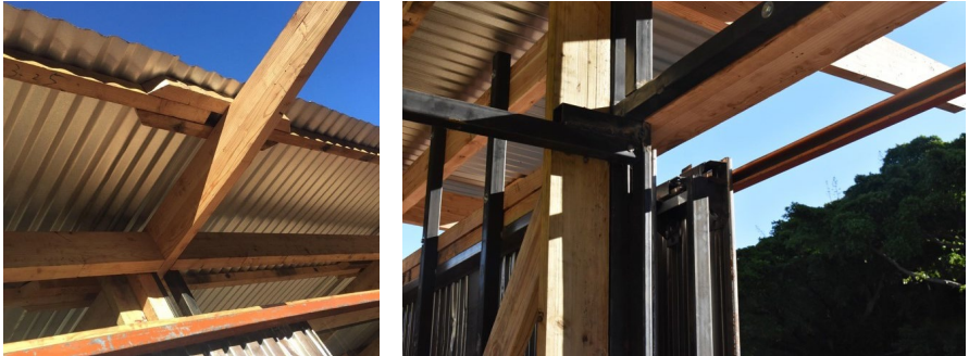
Figure 2. Purlin joint and mechanism for the sliding walls from reclaimed stock (Shall 2019).
