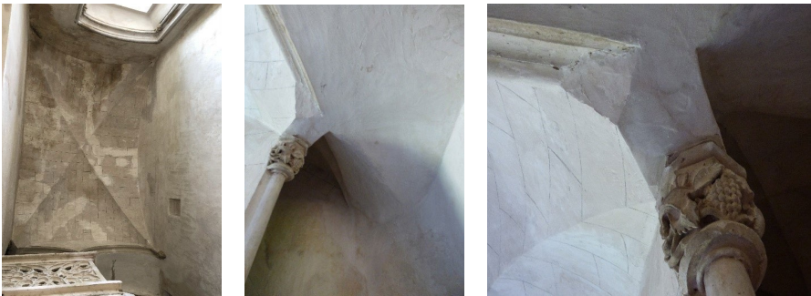
Figure 3. In the first image we see the problem in the outline the upper vault of the stair space whose edges do not coincide at the vertices. The second and third images show problems of joints and geometry posed by the incorporated mullion, originally the top or square post of the flamboyant L-shaped railing, which is strangely extended to form the start of the added ascending staircase. Source: photographs by the author.
