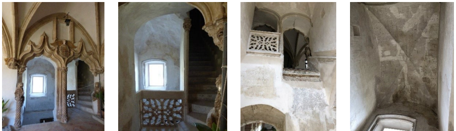
Figure 2. Images of the heritage elements found and cleaned. Source: photographs by the author.
