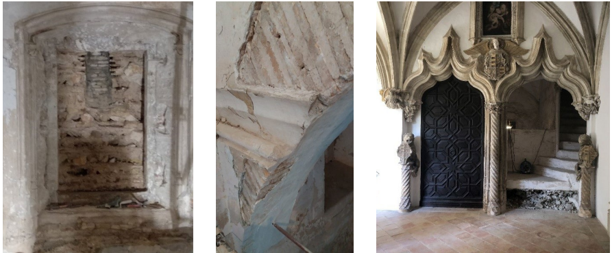
Figure 1. Partitioned façade hole after removing the painting. Springs and carved railings on walls and facade after removing the door, where the overlapped staircase can be appreciated which was later removed to reveal the lower original one. Behind it, the partition on the flamboyant railing. Source: photographs by the author.
