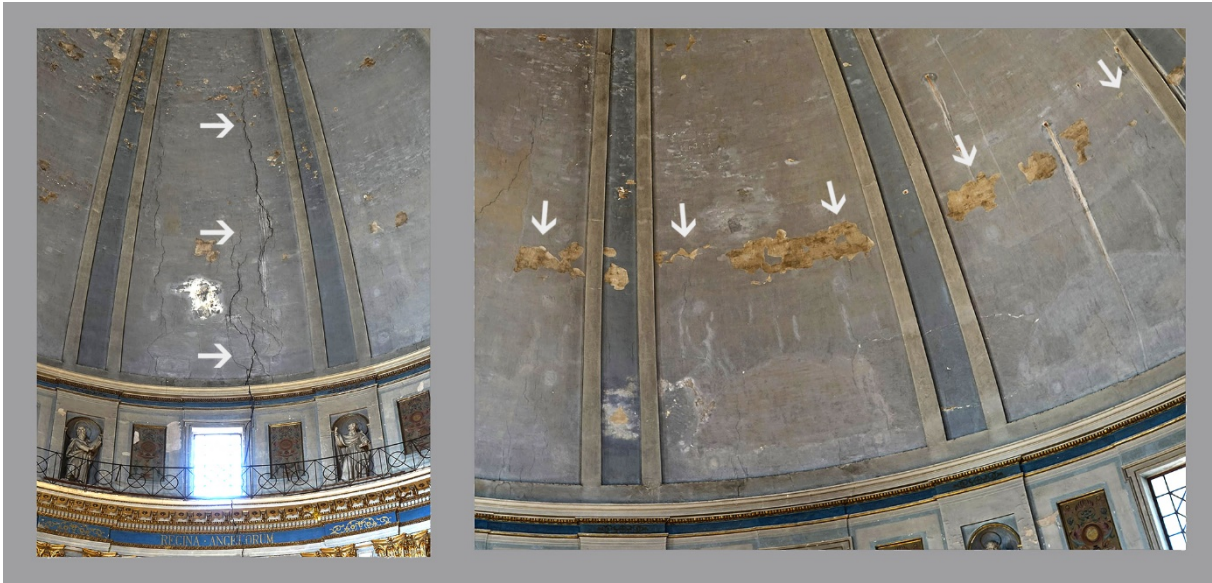
Fig. 8 Dome damage. Meridian cracks (left) and lines of chipping forming a ring (right). Source: Rodríguez-Navarro & Gil-Piqueras
