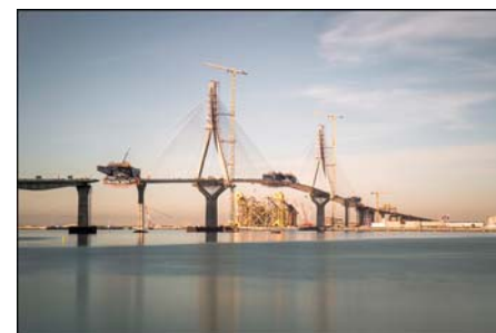
Fig. 16: Cádiz Bay Bridge (2015) in Cádiz, Spain. Main span: 540 m (Spain span length record). Design engineers: J. Manterola, A. Martínez, M.A. Gil Ginés, J. Antonio Navarro, S. García, S. Criado, B. Martínez, L. Blanco, R. González and G. Osborne. (Courtesy of Carlos Fernández Casado S.L.)
