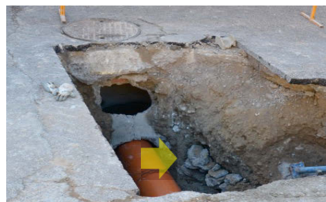
Fig. 6. Supporting the previous argument, it is especially relevant to observe in the two photographs 5 and 6, the holes or highly washed areas that appeared next to the manhole and collector (indicated with an arrow). These have been filled with rubble from the excavation itself, to later proceed to pour the sealing concrete of the connection socket of the new collector with the manhole. These two points would be connected and present a clear continuity parallel to the collector and apparently towards the lower part of the church's street.
