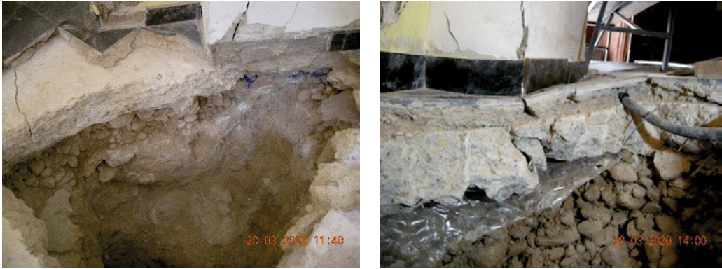
Fig. 7. Pit n°2, (interior). Next to the foundation wall of the Church. The fractured concrete floor and the foundation are recognizable. In the second photograph, detail of the deformations of the floor. Cracks are recognized in the base of the wall due to fundamentally vertical component thrusts.
