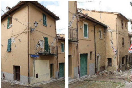
Fig. 1. Terrace in Castelsantangelo sul Nera: damage on head unit (left), overturning of façade in jutting unit (right)
