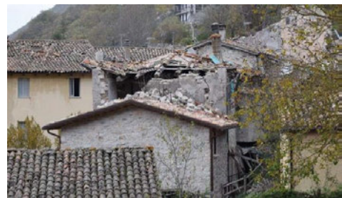
Fig. 3. Overturning of standing walls (Castelsantangelo sul Nera)
