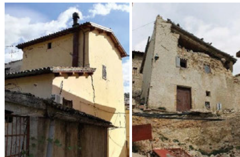
Fig. 5. Left: pounding owing to staggered roofs (Pieve Torina); right: masonry crumbling and r.c. roof collapse (Campi Alto)
