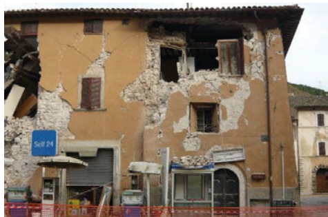
Fig. 4. Crumbling of masonry and shear damage owing to misaligned openings (Visso, courtesy of Eng. Falsetti)
