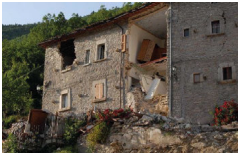
Fig. 2. Overturning of façade in a clogging unit (Noeria)
