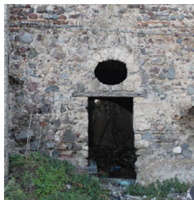
Fig. 5. Fortified house Fasano, detail of the access to ground floor: note the masonry construction 'a cantieri' and the flat-tenting surface of the masonry section using brick elements (Source: Ragosta, 2022).
