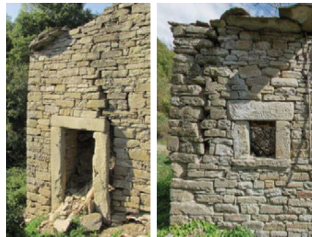
Fig. 7. Vertical bending and overturning mechanisms.
