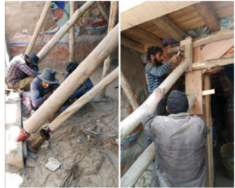
Fig. 15-16. Installation of the props with hydraulic jacks (left). Fixing a temporary load distribution timber frame on the columns and beams (right).
