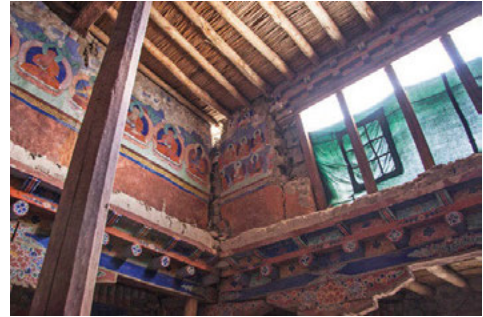
Fig. 7. The severely damaged, tilted, and detached walls on the first floor of the temple's chamber (North-west corner).
