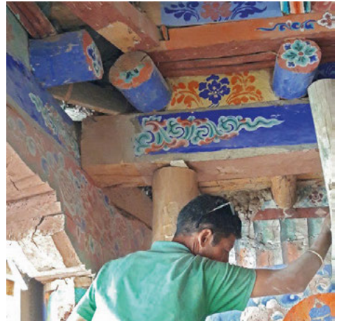
Fig. 11. One of the main beams slid 25cm outside its original position (North-eastern corner).
