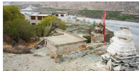
Fig. 1. The dilapidated roof of the Dukhang Yokma (middle ground) and the main monastic complex in the background.
