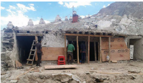
Fig. 14. Installation of plywood panels to temporarily lock the mud brick and stone walls with paintings. In the centre, a series of props are put under the cantilevered poplar beams.
