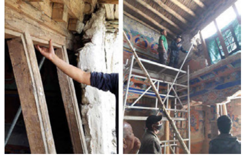
Fig. 10. Tilted wooden opening on the first floor (left); covering the paintings with a protective cloth near the wooden window (right).
