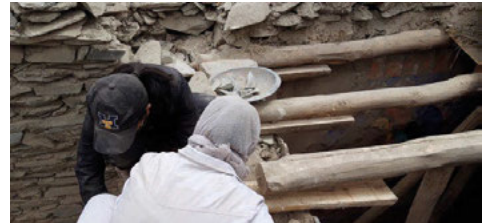
Fig. 17. Placing cantilevers under some of the beams of the entrance hall and fixing them to the stone wall.
