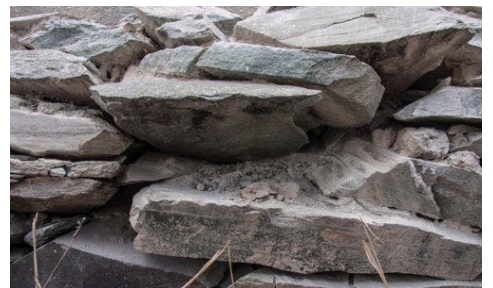
Fig. 5. Bulging plinth with eroded mud mortar (North-east).
