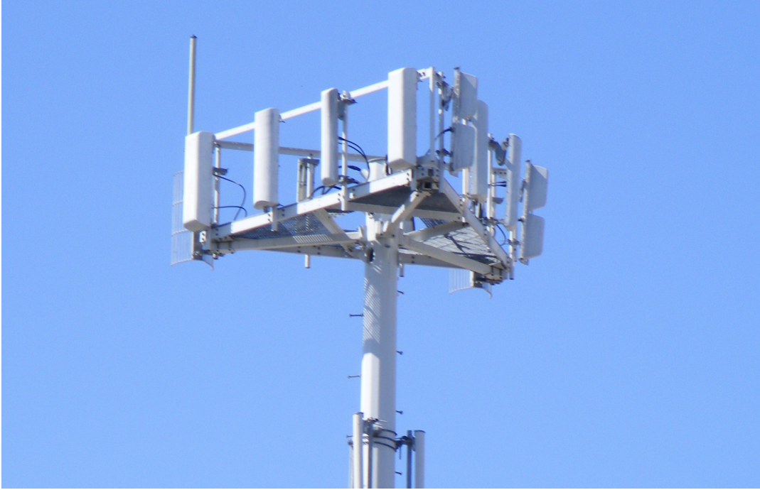
FIGURE 2.21: Cell tower carrying antennas of four cellular networks
