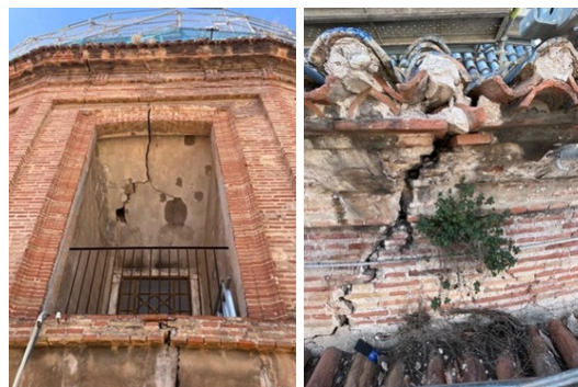
Fig. 2 - Cracks in the lintel and flare of the drum window (left) and in the second ring of the drum where it meets the roof (right).
