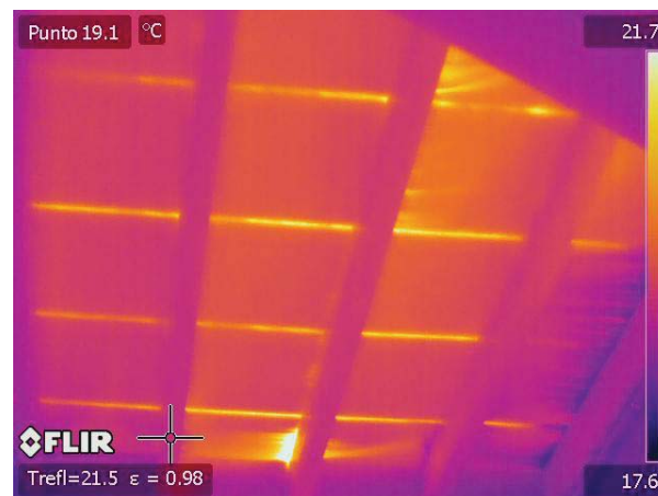
Figure 1. Example of air leakages at the internal side of a rehabilitated roof in an alqueria: cold and hot air leakages.
