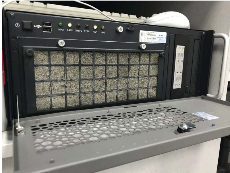
Figure 2. Server computer where the first airflow visualization was detected.
