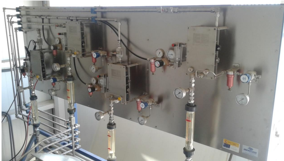
Figure III.14 Error! No bookmark name given.: Photo of the system wall containing four cells for EO treatment of water.
