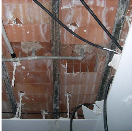
Fig. 1. Joists with the active reinforcement corroded – only the remaining rust can be seen
