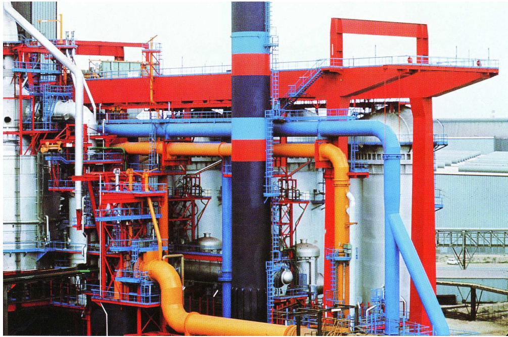
Fig. 31. Solmer Steelworks, Jean Philippe Lenclos, Fos Sur Mer, Marseille (France). In: Linton H. Color in Architecture : Design Methods for Buildings, Interiors, and Urban Spaces. New York & London: Ed. McGraw-Hill, 1999. pp 267. 151x99mm (300 x 300 DPI)
