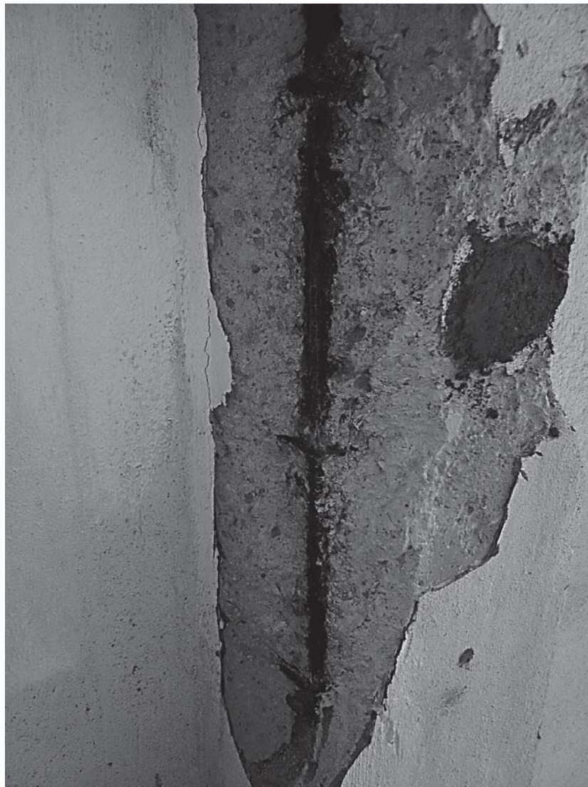
Fig.1. Spalling in cover of column
