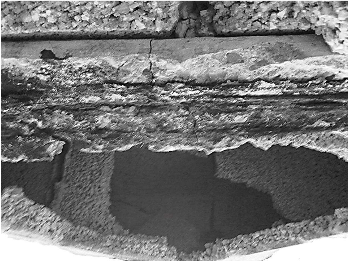
Fig.4. Spalling in joist cover
