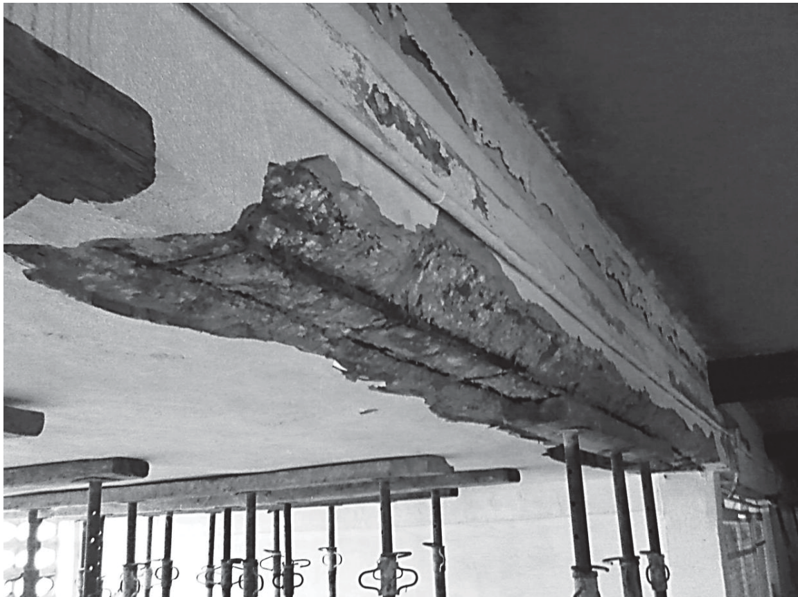
Fig.3. Spalling in beam cover
