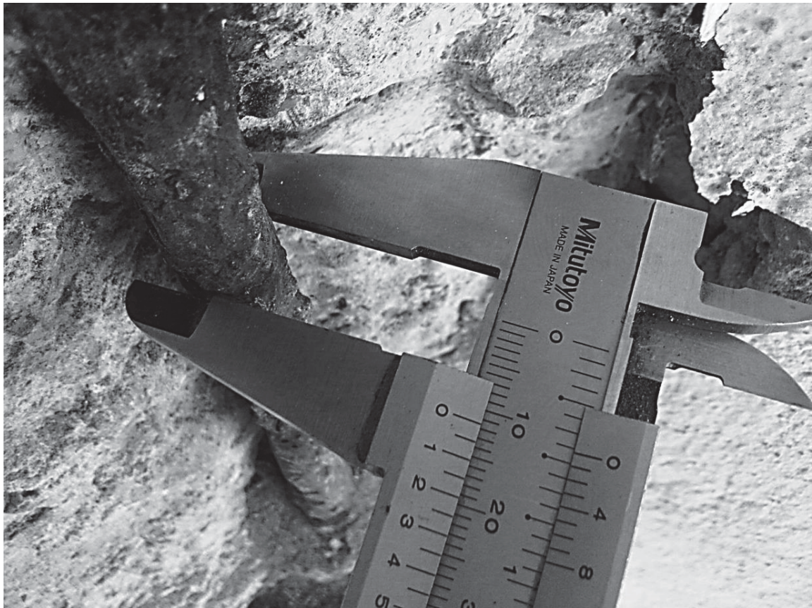
Fig.2. Corroded rebars in column
