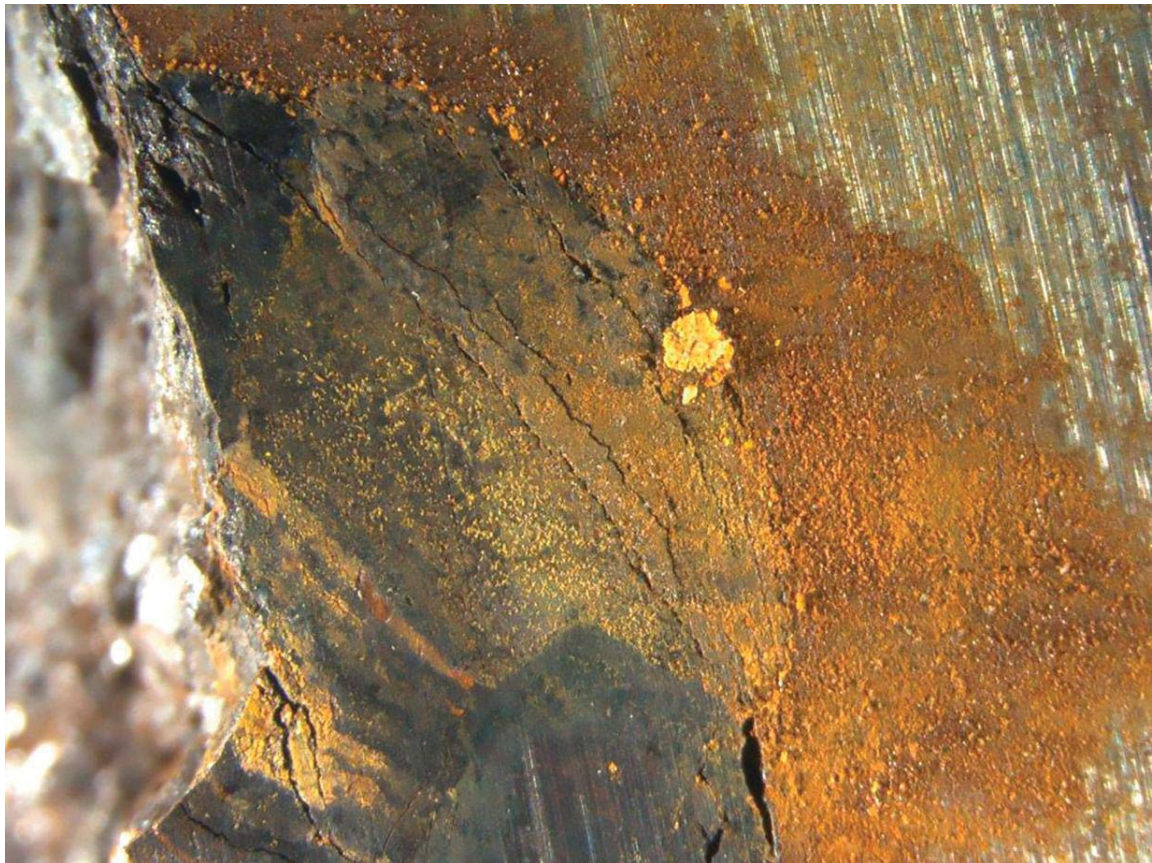
Fig.9. Detail of pitting with a crust of saline particles
