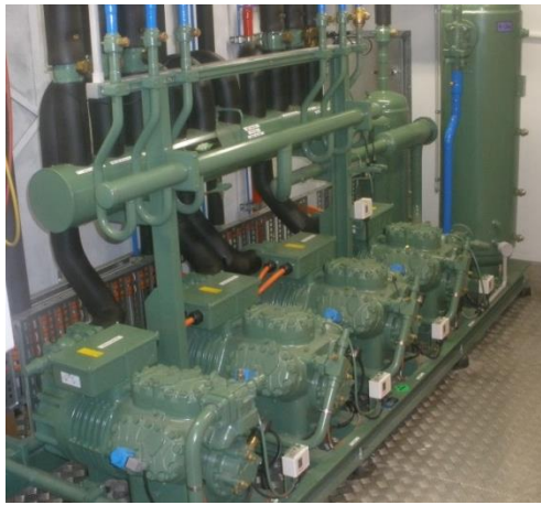
Figure 1. 24. Parallel compressor R134a rack
