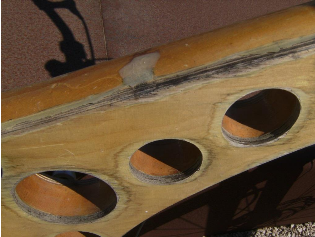
Figure 179. Xylon Hybrid Flaking, Lifting and Weather Damage. Taylor, Nichols. 2015
