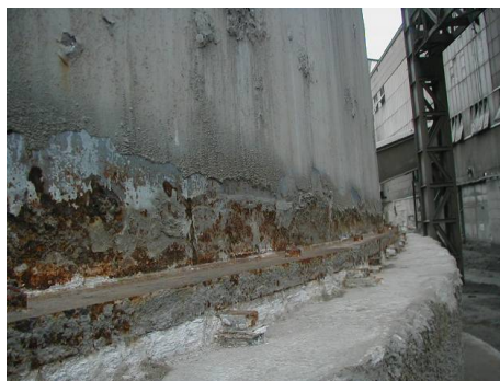
Figure 3: State of the Shell in Contact with the Base Plate
