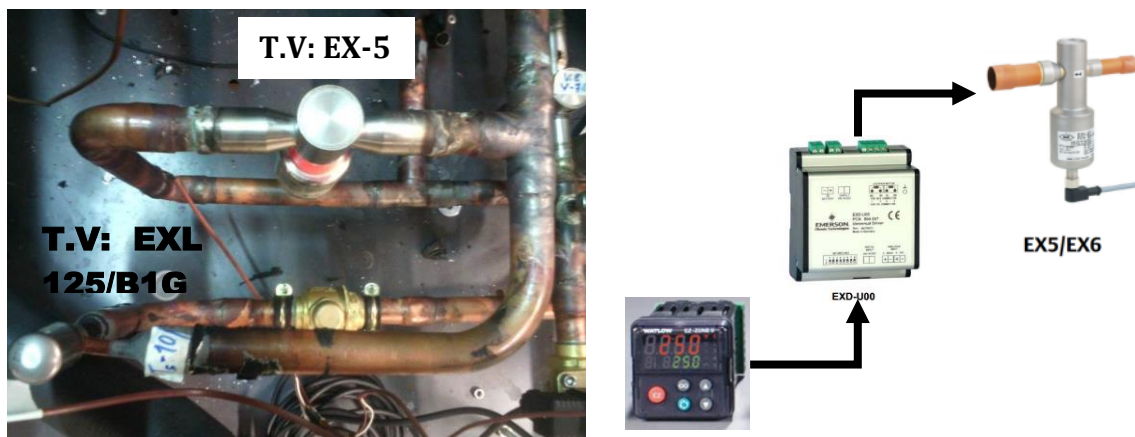
Figure 3.10: Picture of the throttling valves: EX5 and EXL 125/B1G and schematic of the control for the throttling valve: PID → EXD-U00 → EX5
