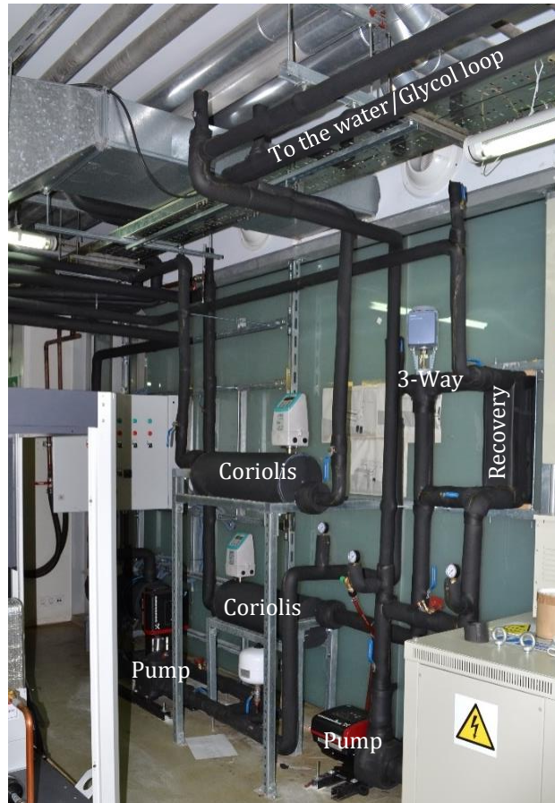
Figure 4.4: Picture of the evaporator and condenser water loop in the test rig
