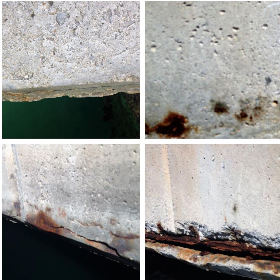
Figure 7.5: Photos of the corrosion rate matching the four indications
