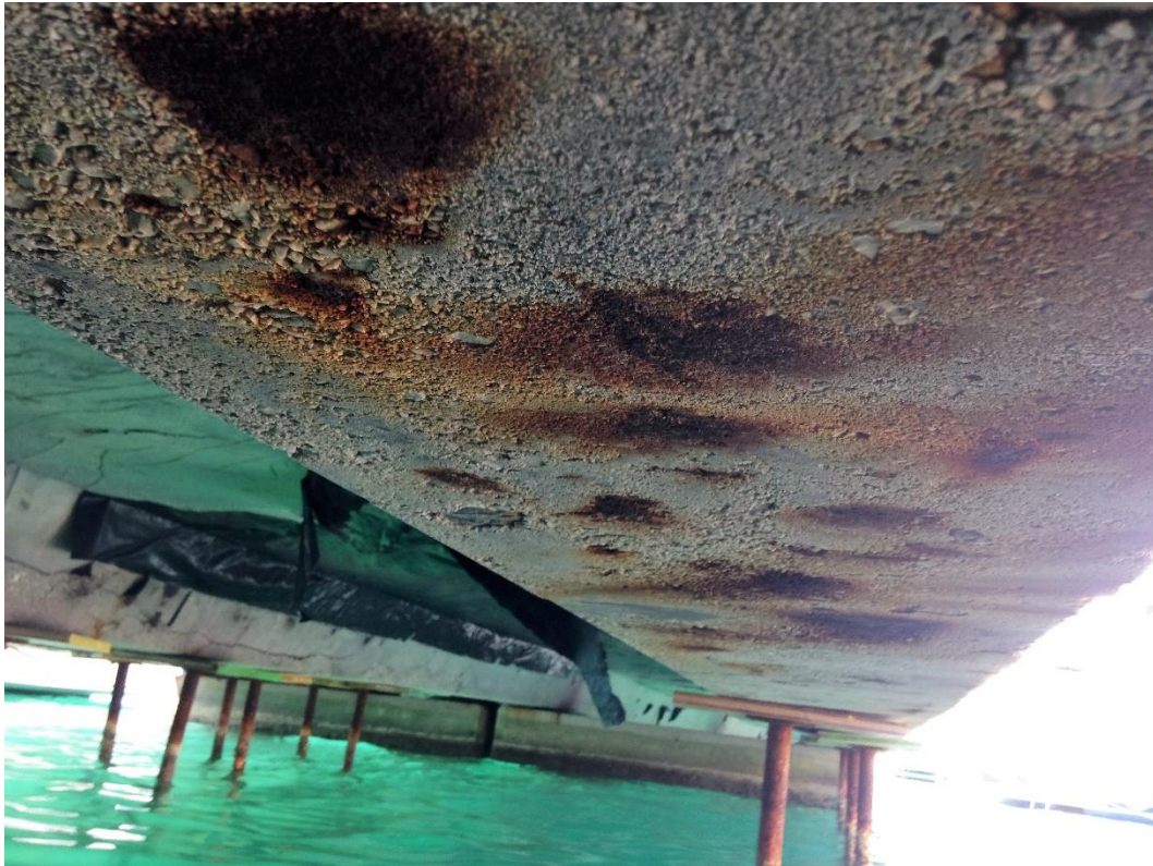
Figure 7.6: Photos of the current state of the downside of the pontoons
