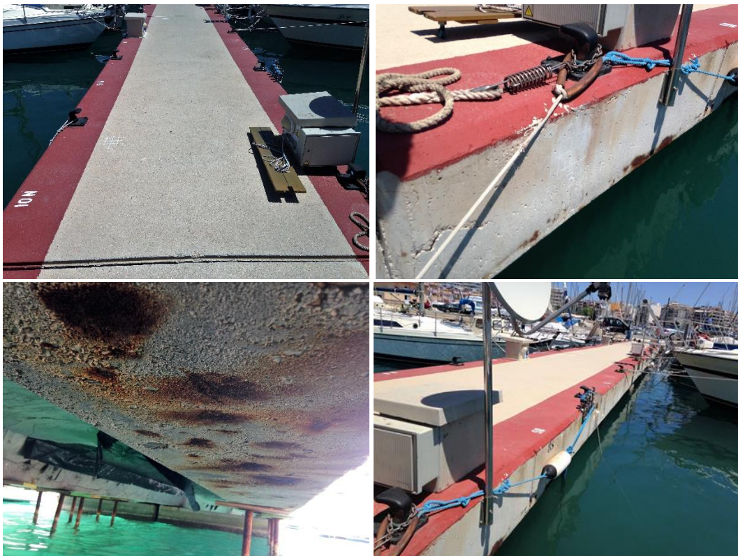
Figure 8.1: Photos of the different surfaces of the deteriorated slabs
