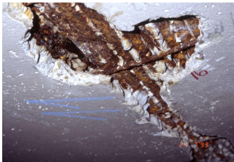
Fig 3.1: Concrete affected by corrosion (Portland Cement Association, 2002)
