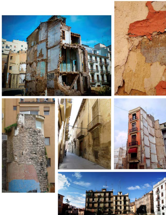
Fig. 2. Urban and architectural degradation in Valencia.
