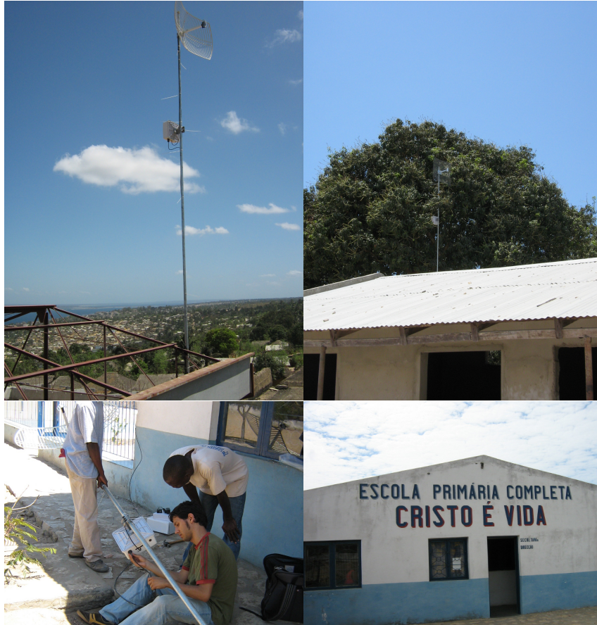
Figure 4.26: In order: An antenna deployed for RuralNet (left up), another antenna (right up), one of our members installing an access point (left bottom), one of the schools of the project (right bottom).
