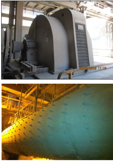
Fig. 3 Photographs of the field WRIM (12P, 3.3kV, 1,500 kW) and of the driven mill.
