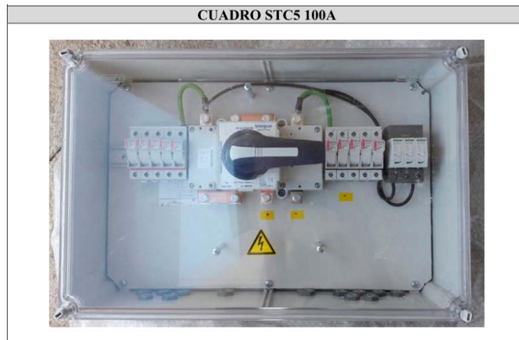
Figure 11. Junction box of a maximum of 100 A (provided by manufacturer AMB Greenpower).
