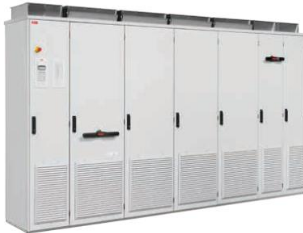
Figure 7. Detail of the central inverter (provided by manufacturer ABB).
