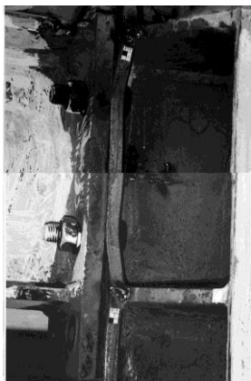
Fig. 8. Brittle cyclic failure of bolts in sagging for an end-plate connection [17].
