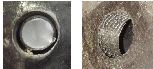
Fig. 16. Observed damages (P15.1-1)
