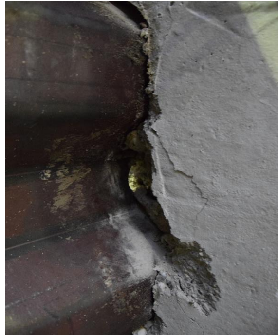
Fig. 9. Concrete crumbling at the web-to-slab connection (P17-T-14).
