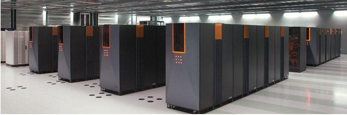
Figure 4. Data centers are the main target for the implementation of the L3 MATRIX devices. (http://l3matrix.eu/)
