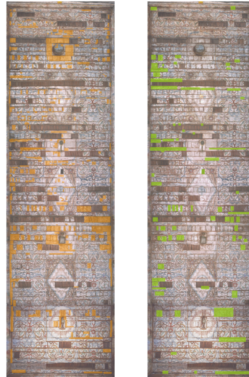
Figure 11:4. General view of the nave ceiling showing the paint losses (orange) and the humidity stains (green). (Photo: Salvador Avila, 2003. Design: K. Muñoz Alcocer, 2004).
