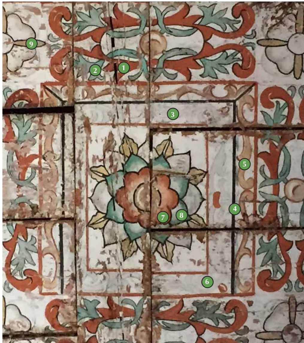
Figure 11:19. Narthex ceiling. View of the studied area and location of the analysed points. (Photo: K. Muñoz Alcocer, 2015; design: Lucia Capitani, 2018).
