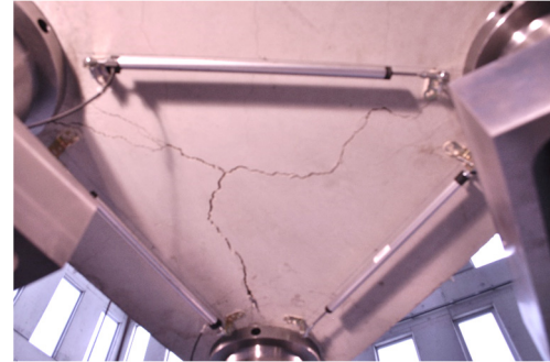
CARA INF – Colapso
