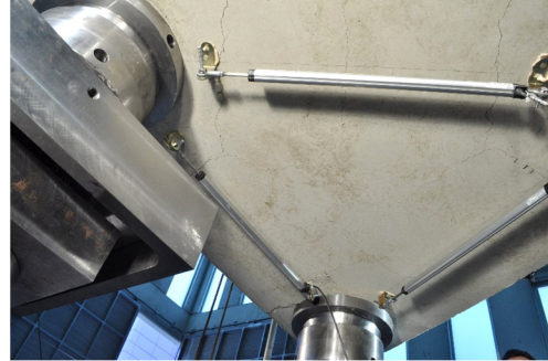
CARA INF – Colapso
