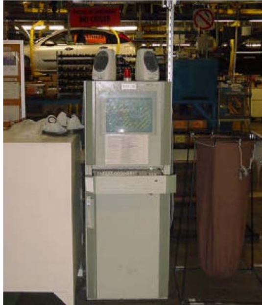
Fig. 5.2 Armario terminal Error Proofing
