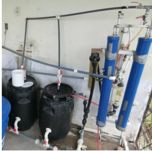
Figure 4. UF plant set up in La Granja (Ecuador)
