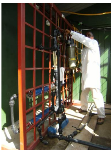
Figure 6. UF plant installed at the Escola Primaria of Ressano García (Mozambique)
