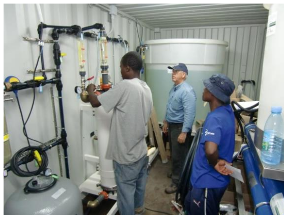
Figure 7. UF plant installed at the Health Centre of Ressano García (Mozambique)
