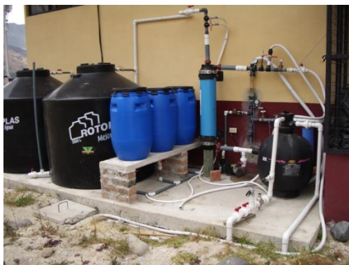
Figure 2. UF plant set up in Girón (Ecuador)
